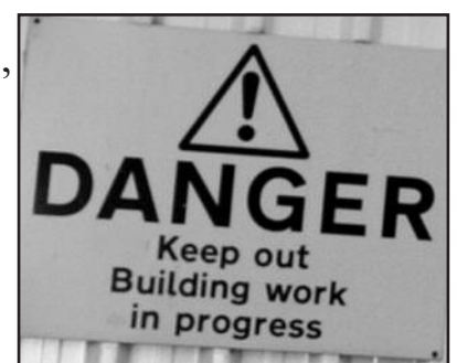
Right: Danger says it all. Sign outside the Mansion warning the public that the site is still very much a danger. No sign, though, of when it will stop being dangerous to the public and re-open.
